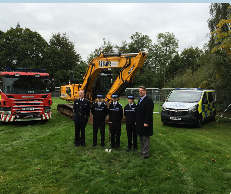
Turf cutting ceremony for the new joint police and fire Operations Communications Centre at Hindlip
